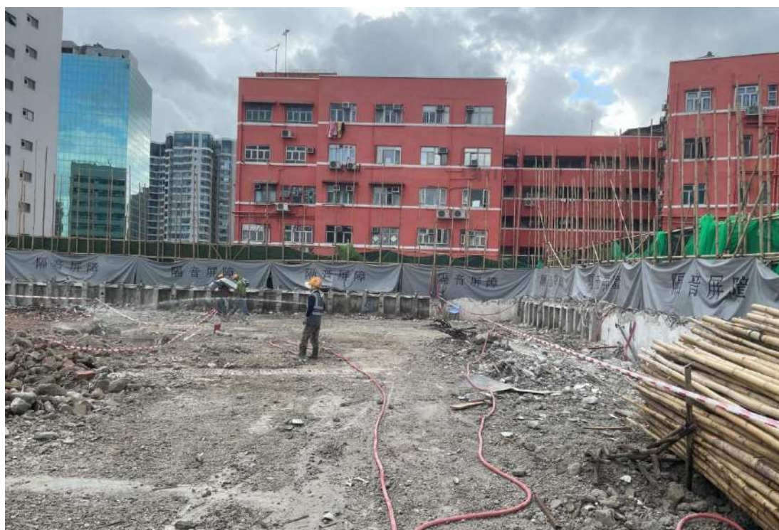
Figure A1: Properly erected noise barrier mat surrounding 4 sides of the building
